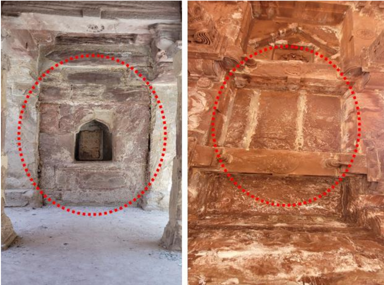
Figure 18: Different layers of stone is visible due to exposure to weathering
