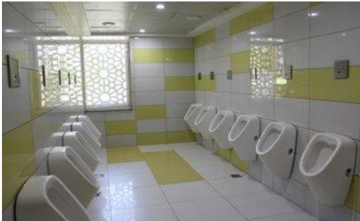
Picture1: Sensor based toilets at MUJ campus
